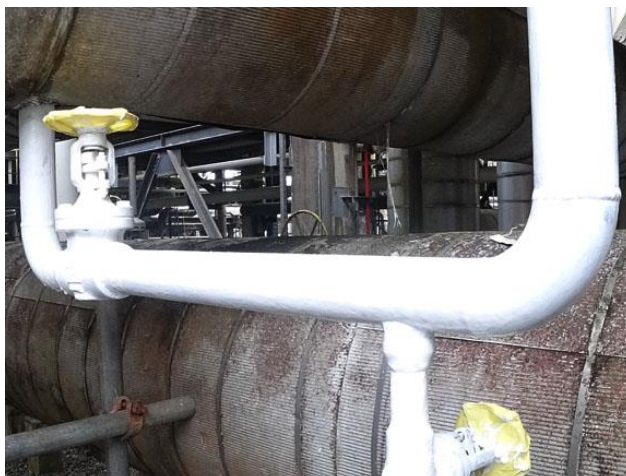
Coating applied during cold surface temperature
