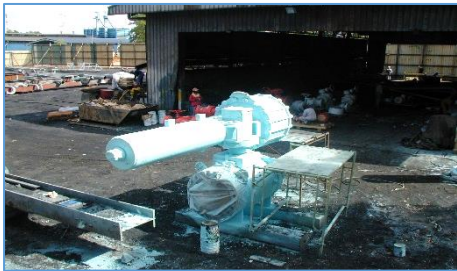
SDV after wet application and all but the flange castings are completed. The flange covers were to be fitted offshore, after installation of the valve.
